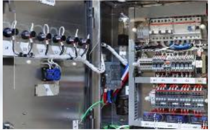
Electric Control Panel
